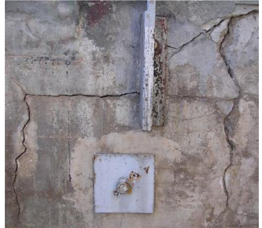
Damages due to the ASR at macroscopic scale
