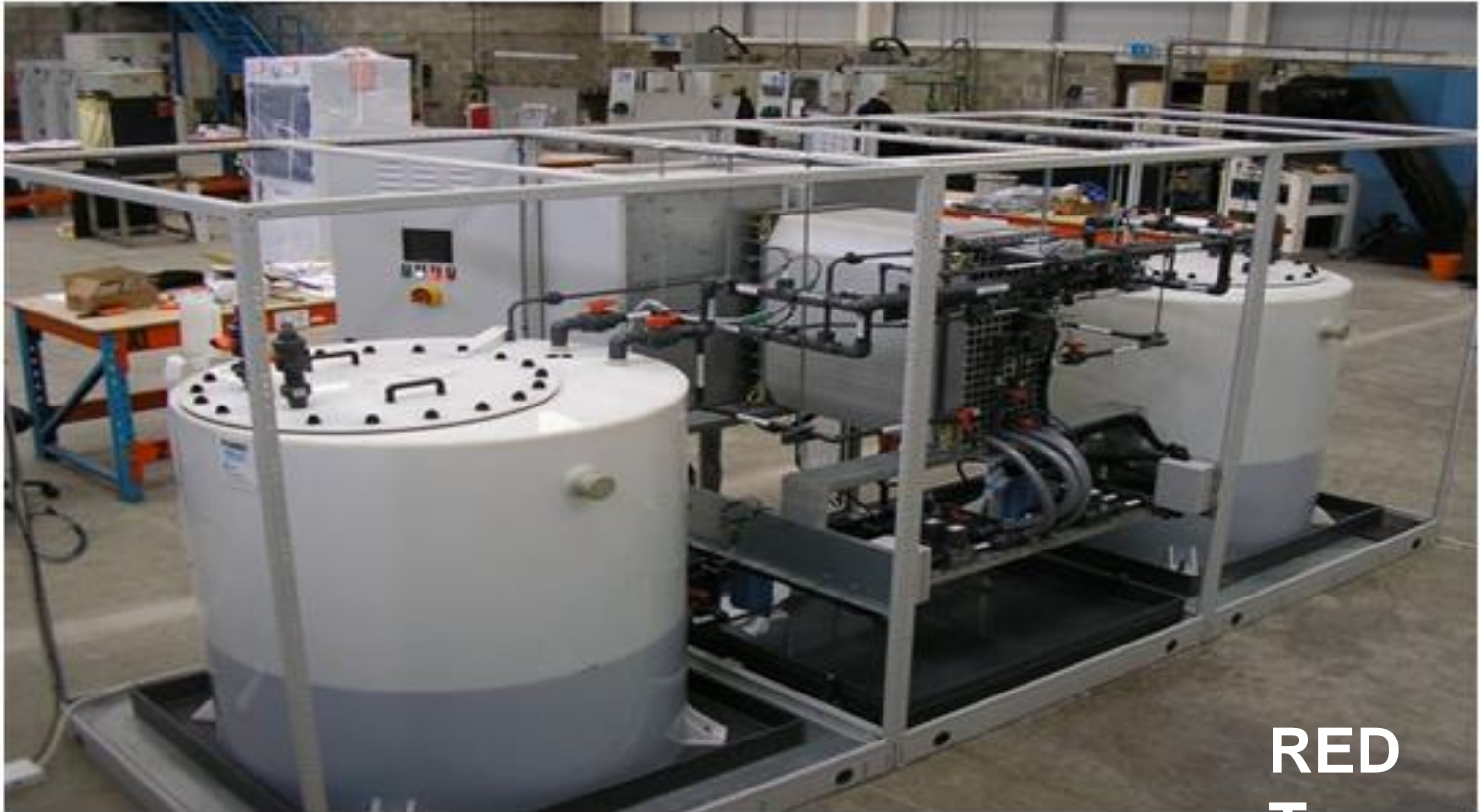
Original 30kWh VRFB pilot system
